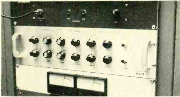
All those knobs belong to the Antlitzer, a unique type of modulation controller which keeps WFMT's signal legal.
